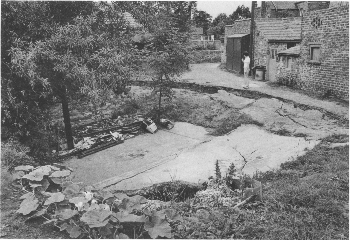
FIG. 2. Subsidence hollow formed on 28th July 1979 behind houses on Magdalen's Road, Ripon (SE 3170 7129), 200 m SE of the site discussed. The garages which stood on the concrete slab had long shown signs of distress and were demolished prior to this catastrophic collapse (photo: Acrill Newspapers).
